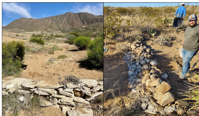
Sul Ross State University and BRI researchers and students constructed 130 trincheras at a private property in Brewster County. To measure soil capture, rebar posts were placed upstream and downstream from 50 of these trincheras. Significant soil accumulation was shown to occur upstream of the trincheras, and minimal soil loss occurred downstream.
